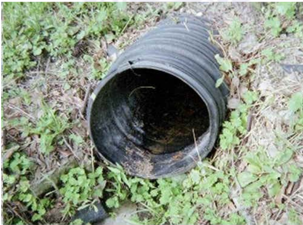
FIGURE 3. CLOSE-UP OF INSIDE PIPE OF FIGURE 2. STANDING WATER INSIDE A "DRAINAGE" PIPE. UPTURNED END OF PIPE EITHER DUE TO IMPROPER INSTALLATION OR KNOCKED UP BY CAR GOING INTO DITCH. ANOTHER UNNECESSARY MOSQUITO-BREEDING SITE.
