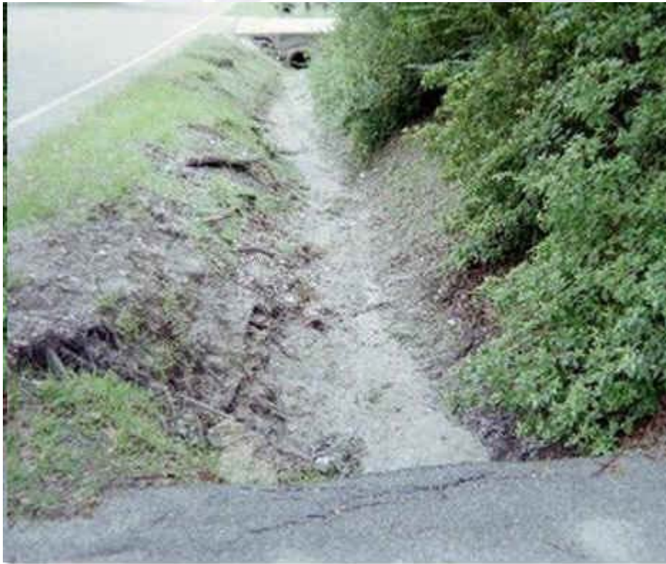
FIGURE 4. A CORRECTLY DONE DRAINAGE DITCH. NOTE SAND IN BOTTOM WHICH CAN SHIFT TO FILL LOW SPOTS. NOTE NO STANDING WATER IN DITCH OR AROUND PIPES UNDER DRIVEWAYS.
