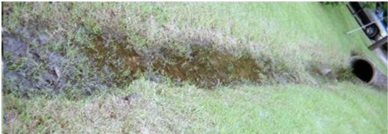
FIGURE 1. STANDING WATER IN A DITCH THAT WAS DUG OUT TOO DEEP. NOTE GRASS AND OTHER PLANTS GROWING IN WATER, WHICH MEANS THIS AREA HAS HAD STANDING WATER FOR A LONG TIME. A PRIME MOSQUITO-BREEDING SITE AND HEALTH THREAT TO HUMANS.
