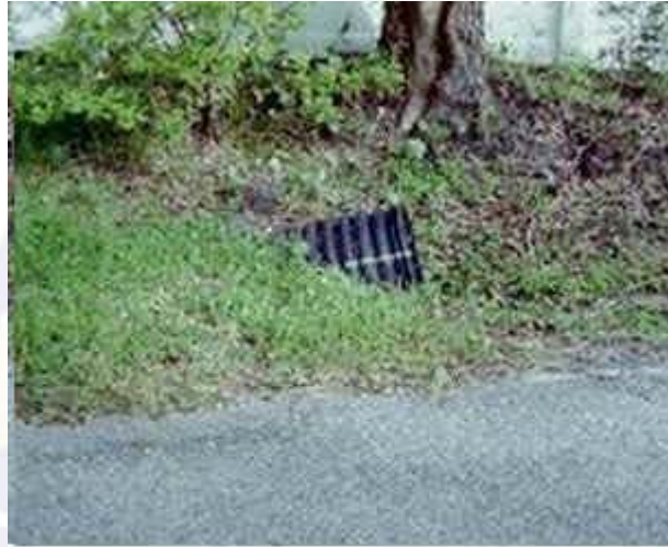
FIGURE 2. SIDE VIEW SHOWING PIPE WITH AN UPTURNED END, CAUSING WATER TO BE RETAINED IN PIPE, LEADING TO MOSQUITO-BREEDING SITE INSIDE PIPE.
